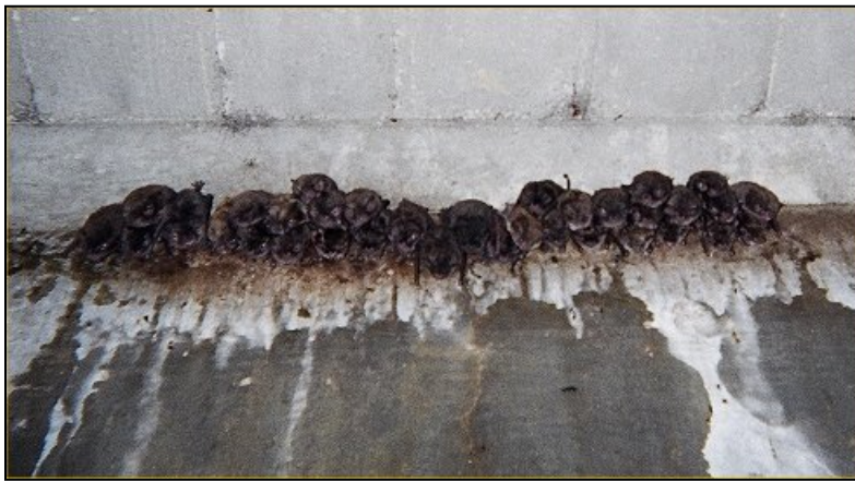
Photo 11: Bats Roosting & Associated Staining
