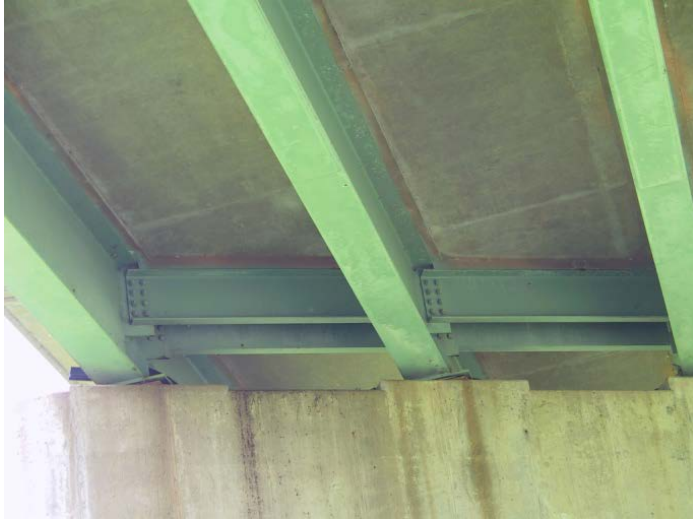
Photo 10: Guano staining on side of pier
